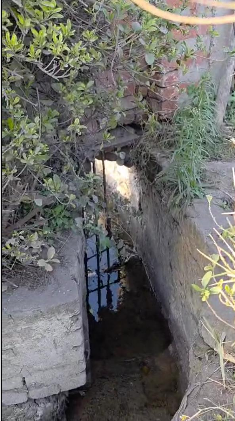
Final outlet going into Dhandera Drain
