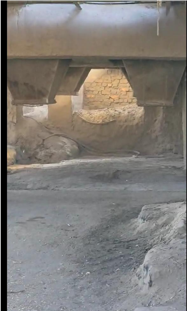
Ash collection point. Found cleaned.
