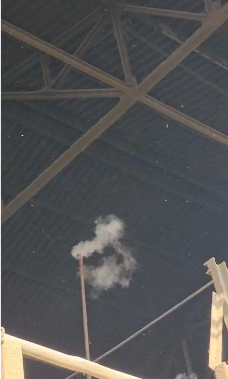
Light weight bagasse particles flying around boiler
