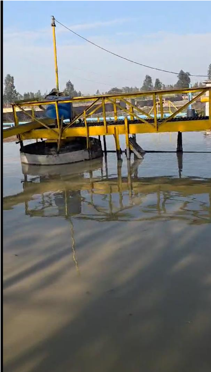
After equalisation the effluent reaches Primary Clarifier
