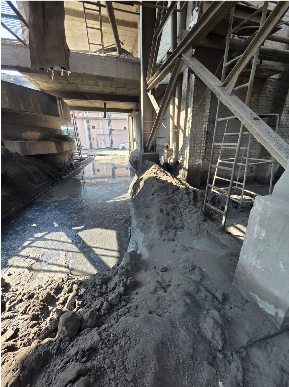
The fly ash collection point was found cleaned with water.
