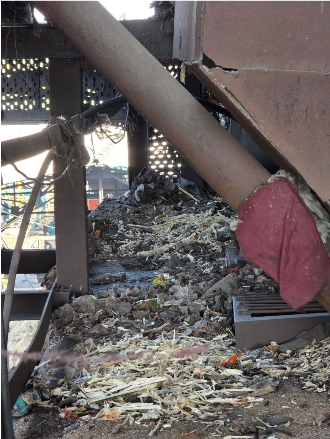
Near the Boiler ↑
