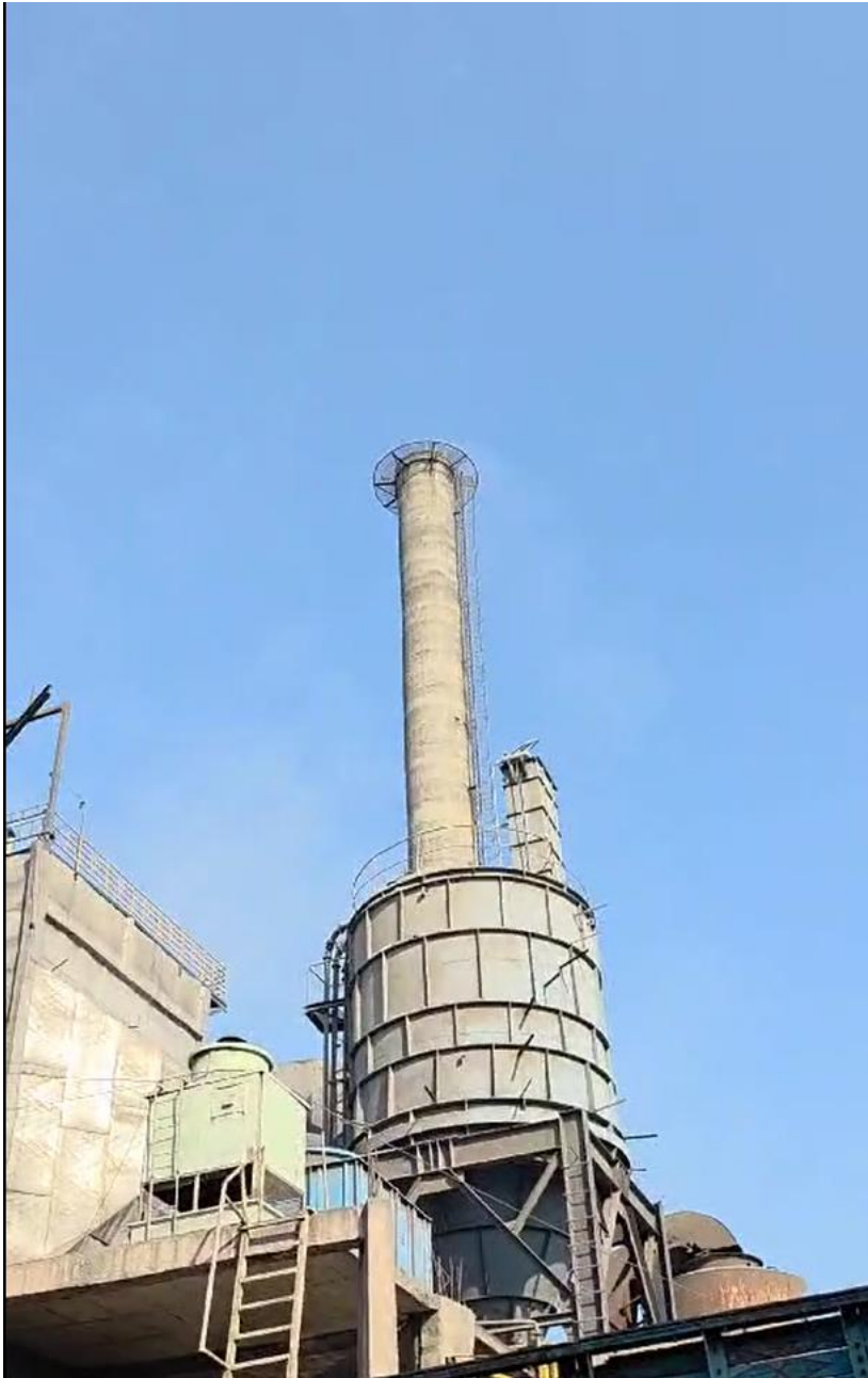
Stack of Boiler
