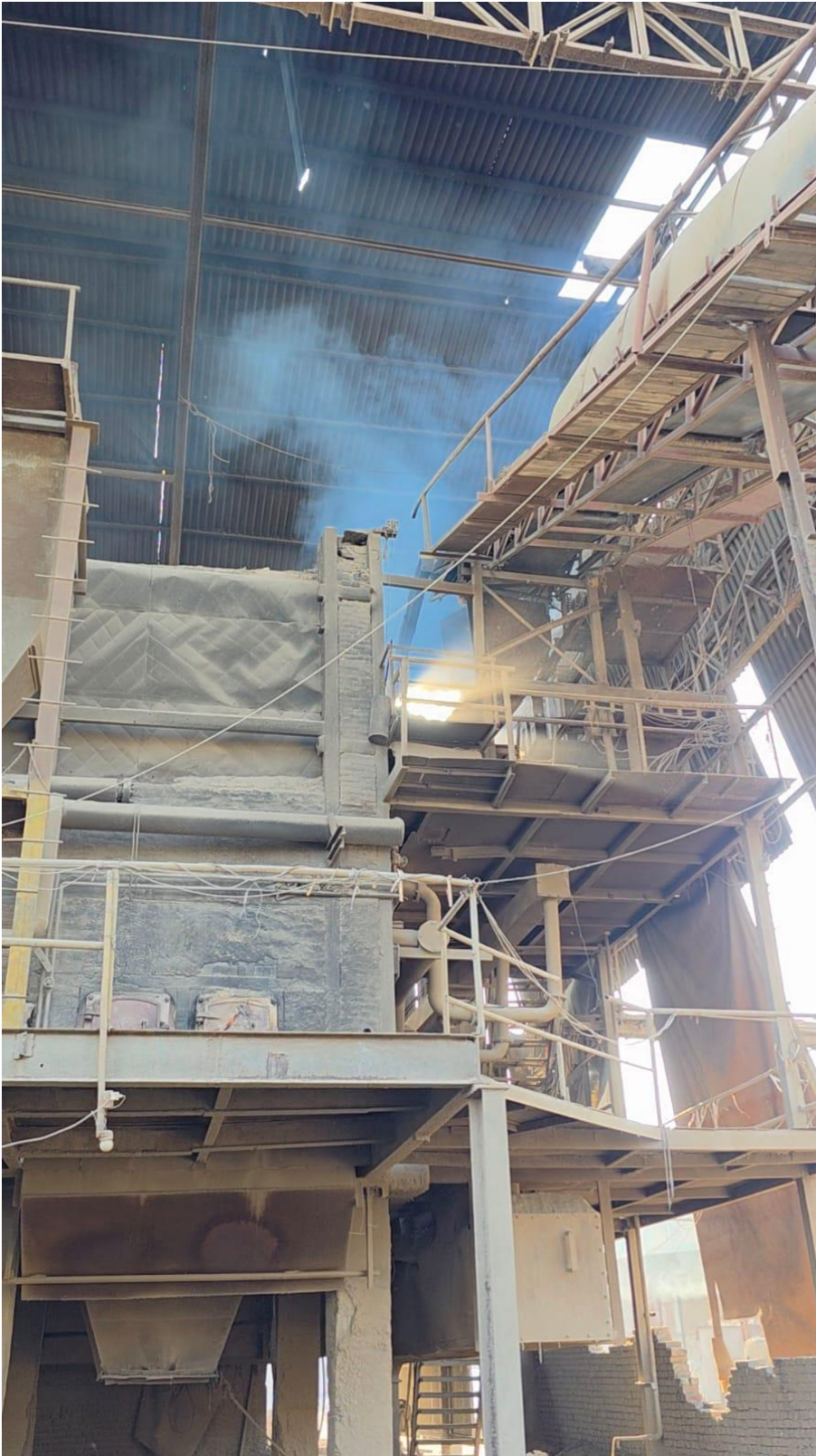
Boiler emitting smoke
