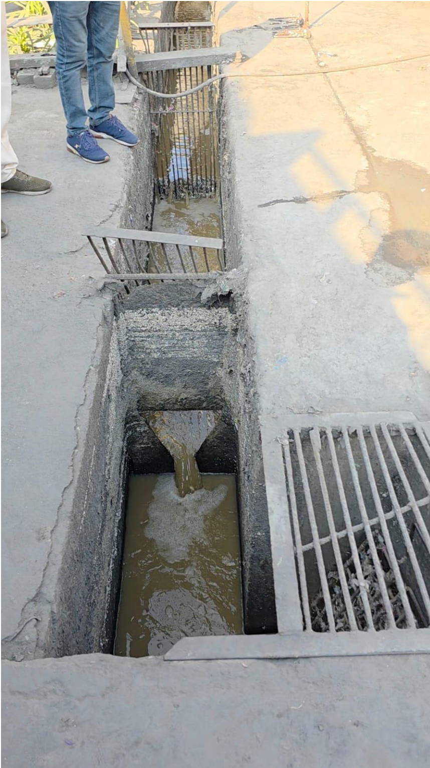
Inlet of unit-1.
