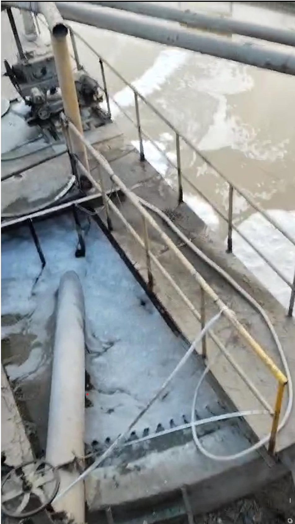
From sedicell the waste water reaches Primary Clarifier.
