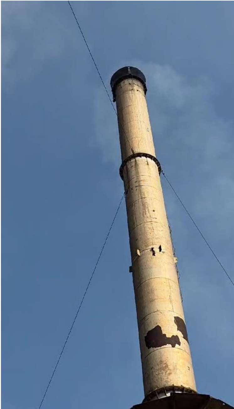
Stack of Boiler
