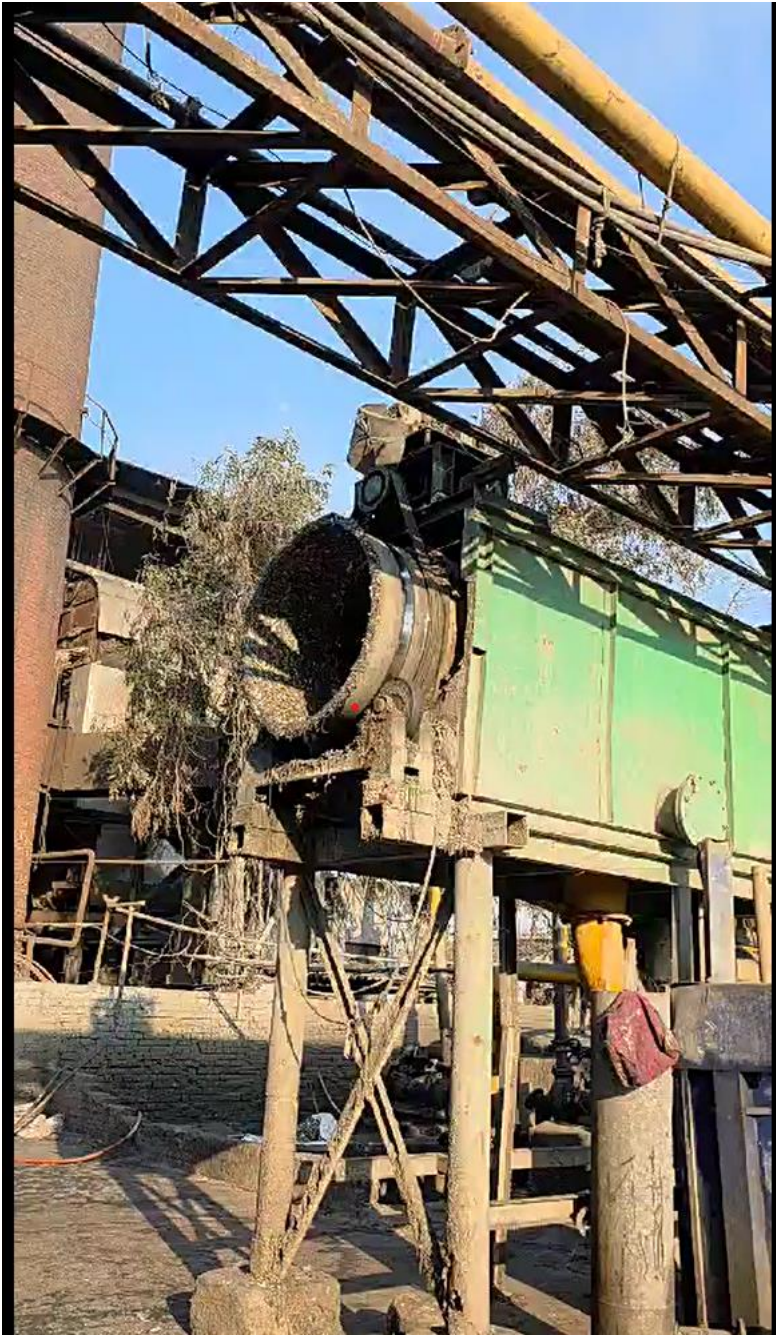
B2 Thickner- used to separate plastic waste from the effluent.
