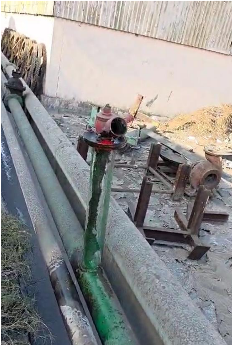
Installed above drain carrying effluent towards ETP of Unit II
